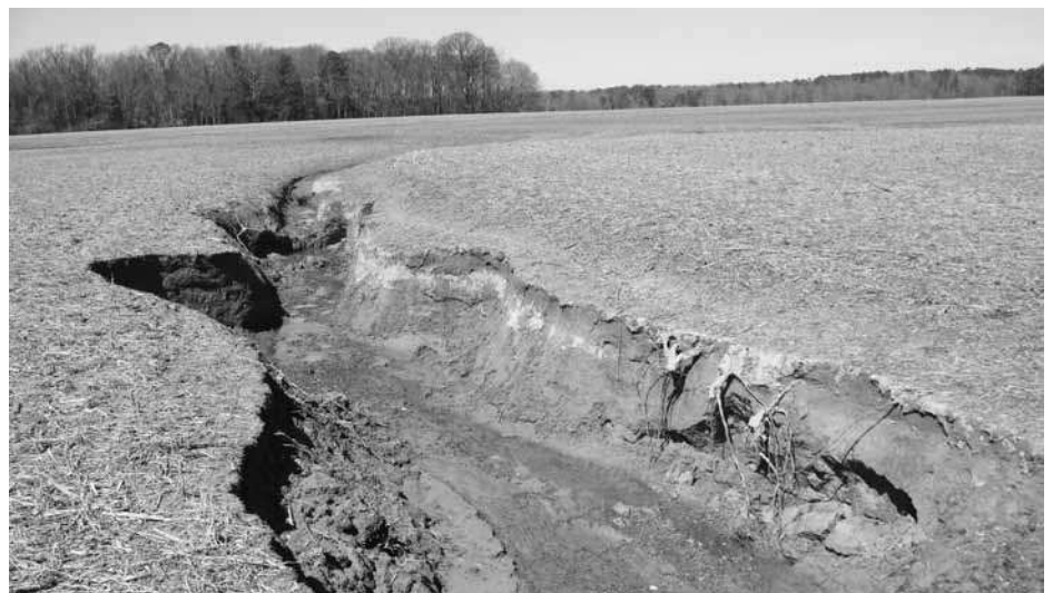
Before: Significant gully erosion in a field at Talisman Farm.
